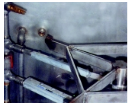
EXAIR air saving blowoff products for drying are installed in a parts washer.
