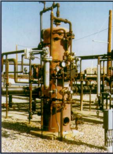
BEFORE: A process vessel with three float switches, two short sight glasses, a pneumatic level controller and 15 valves and associated plumbing.
